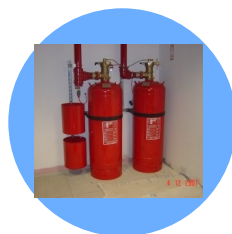
Fire / Gas Suppression Systems
